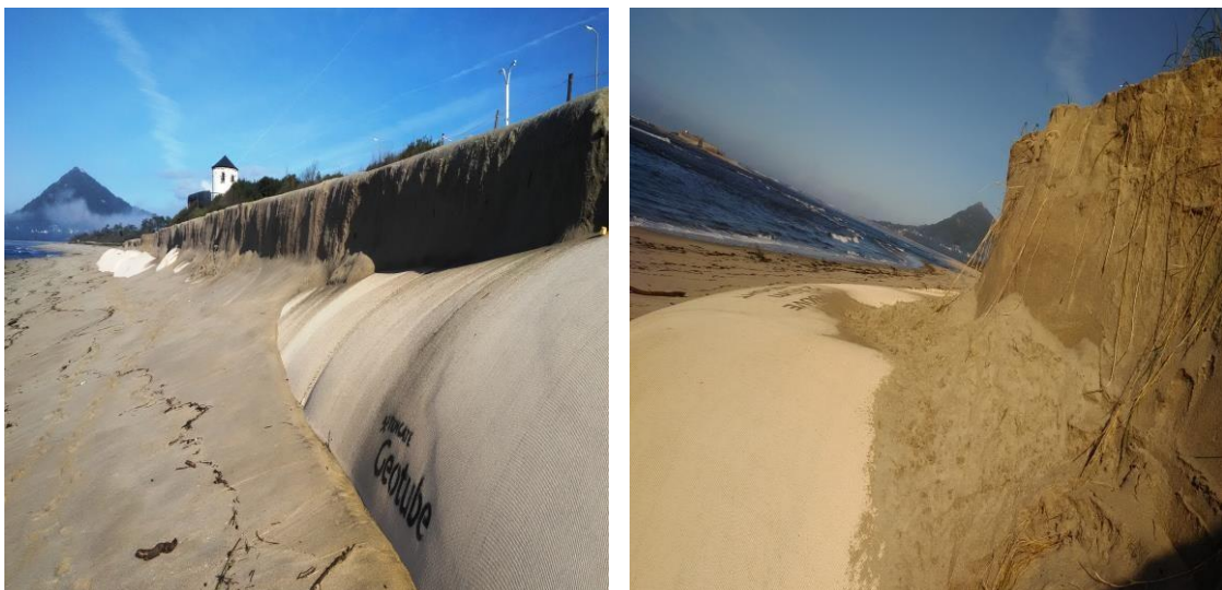
Figure 10 - Moledo beach dune after a storm in December 2019, with dune erosion and exposed geotextile.
